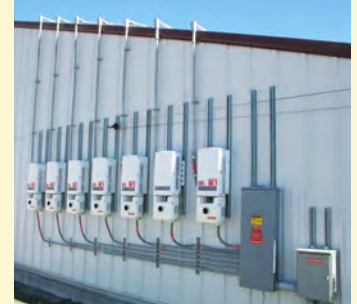
▲ A set of string inverters
