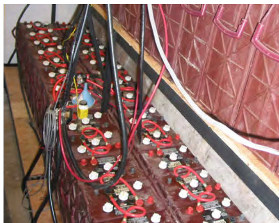
▲ A battery bank
