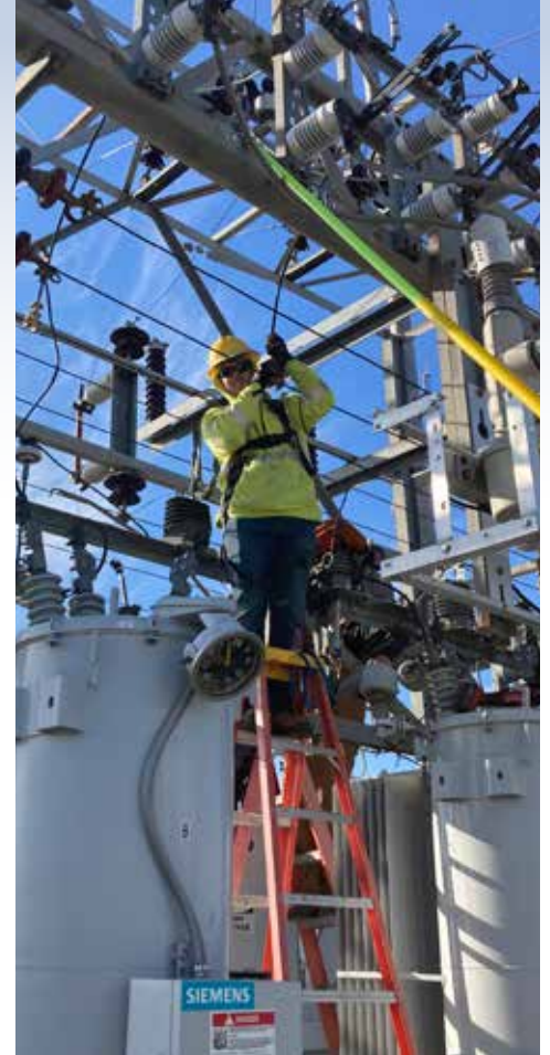
Lineworker Brooks Erickson makes repairs at the Homer substation in Benton County.
